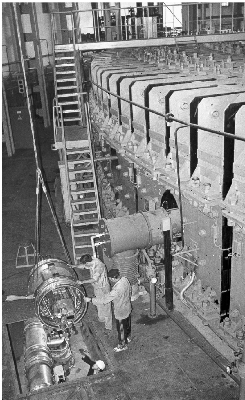
Laboratory of High Energies. Completion of the assembly of the Nuclotron ring's area with elements of the beam slow extraction system
