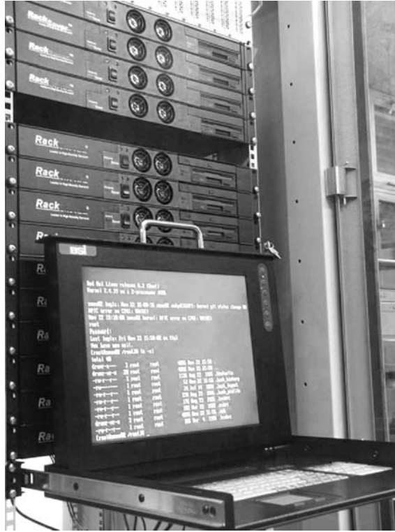
Fig. 4. Tier 2 LCG-1 cluster at ACC Cyfronet, Cracow, consisting of a set of dual Xeon 2.4 GHz processors, connected via 100 MBit/s Ethernet, with a 1 GBit/s uplink
