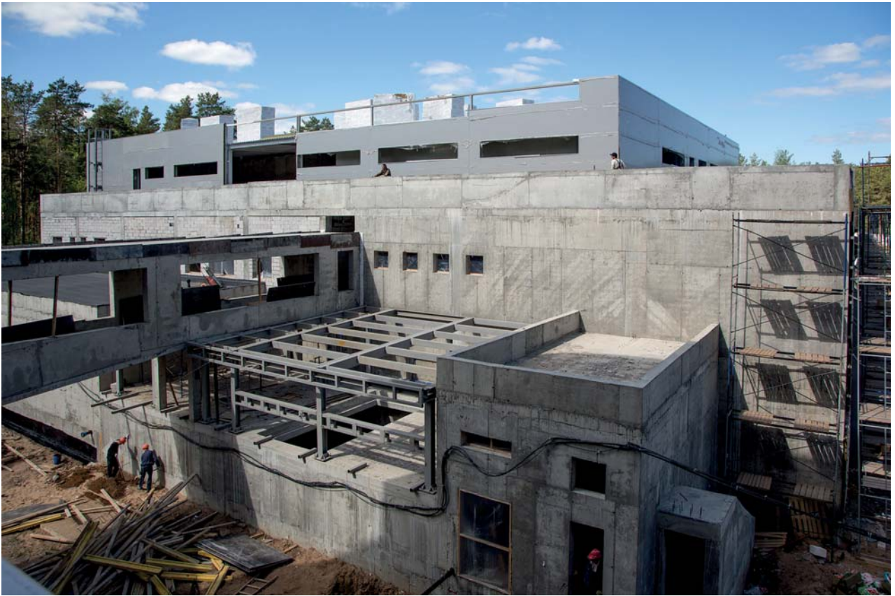
The Flerov Laboratory of Nuclear Reactions. The construction of the Factory of Superheavy Elements
