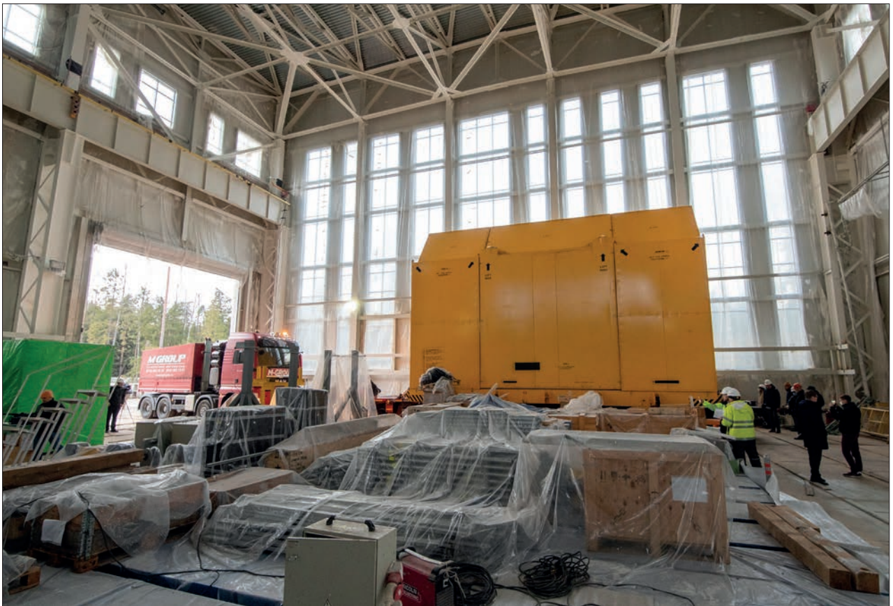
Dubna, 6 November. The superconducting magnet for the MPD detector has been delivered to the construction site of the NICA project
