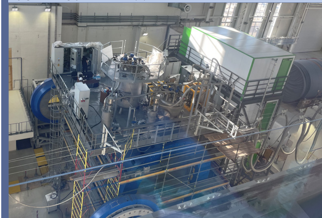
A general view of the technological platform of the MPD solenoid cryogenic cooling system with the equipment installed
