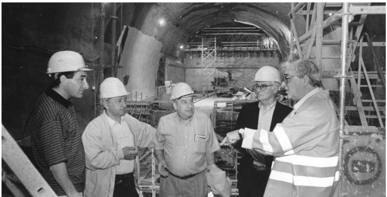
Geneva, CERN. Construction of the tunnel for the Large Hadron Collider continues. JINR's delegation, headed by Vice-Director A.N.Sissakian (second from left), is seen in the LHC cavern on the future site of the ATLAS detector
